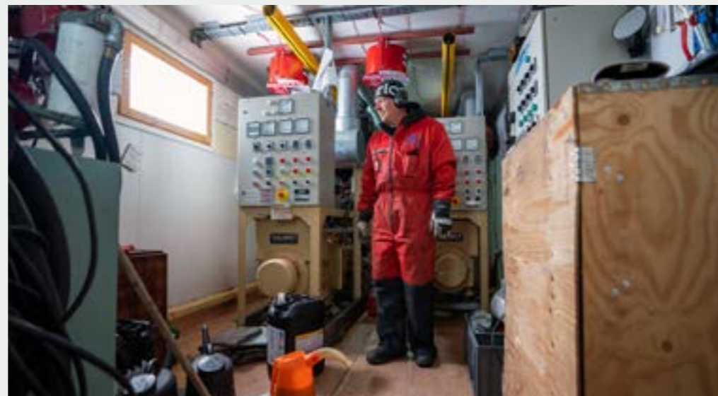
Konemestari mietteisään aseman konehuoneessa. Mechanical engineer in his thoughts at the station engine room.
